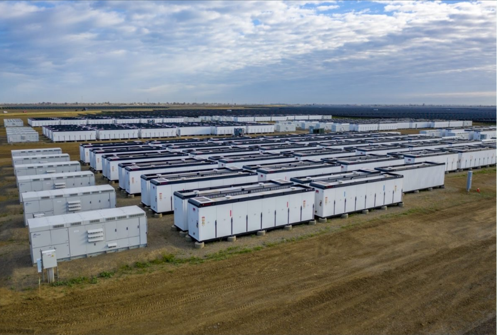
Grid Storage for wind, solar, and load balancing
